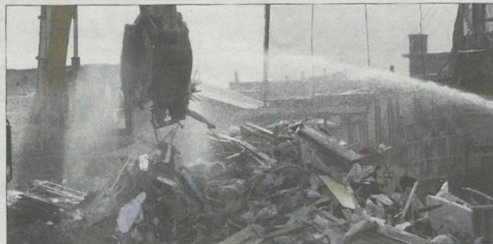
Zeval Transfer LLC is one of the waste-transfer stations in Hunts Point, Bronx. They deal with recycled materials. BESS ADLER
